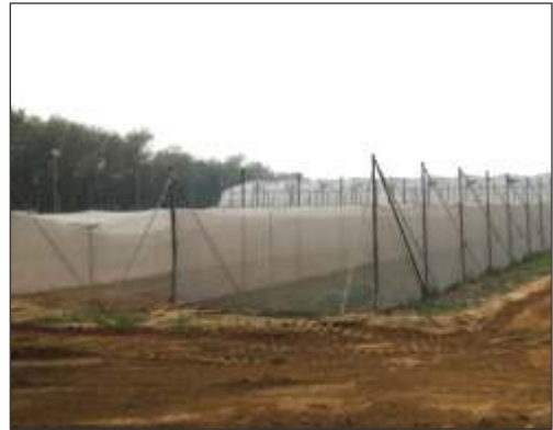
Rectangular shaped permanent insect proof net house with provision of net on the top
